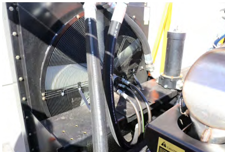
Figure 4: Hydraulic Oil Heat Exchanger
